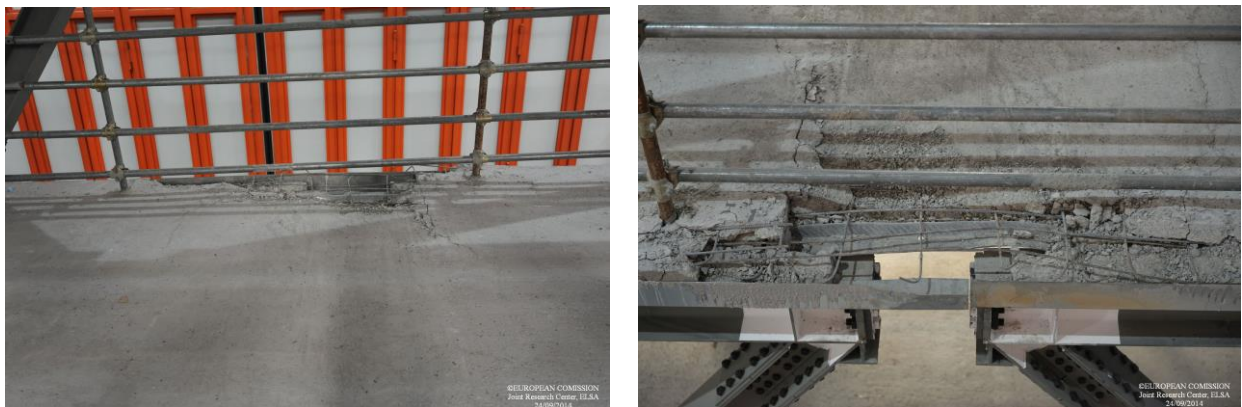
Figure 85. Damaged slab, 2nd floor
