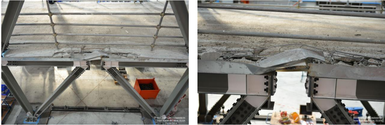
Figure 84. Damaged slab, 1st floor
