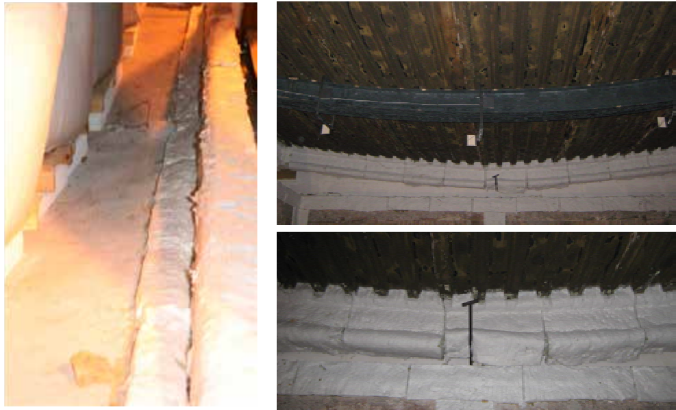
Figure 7.37 Collapse of edge beam
