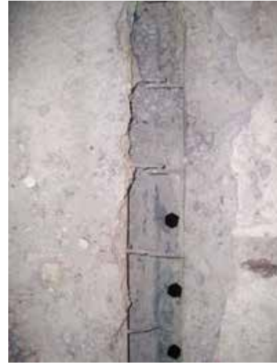
(b) State of the reinforcement joint at the location of the crack after cooling
