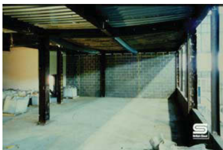
Deformed state of the heated part of the composite floor
