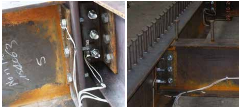
(a) Beam to column joints with flexible end plates and double angle web cleats (b) Beam to beam joints with double angle web cleats
