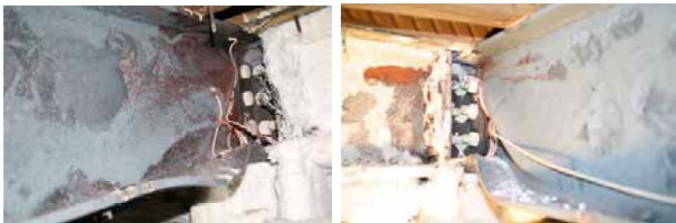
Figure 7.39 Local buckling of unprotected secondary beams
