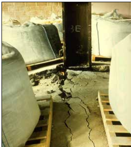
Figure 2.21 Cracked floor slab in region of non-overlapped mesh
