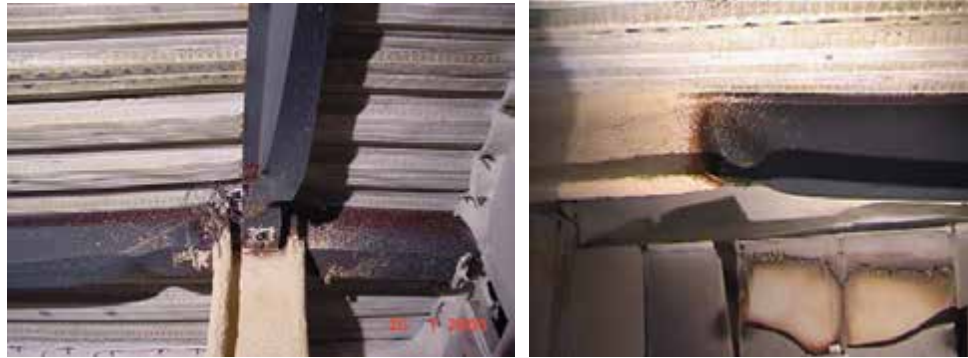
Figure 2.26 Various deformed steel beams
