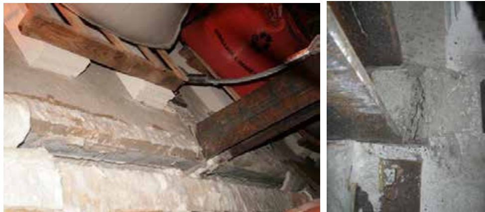
Figure 7.42 Cracking of concrete around central columns
