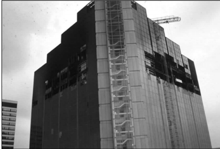
Figure 4.3 Churchill Plaza, Basingstoke following the fire
