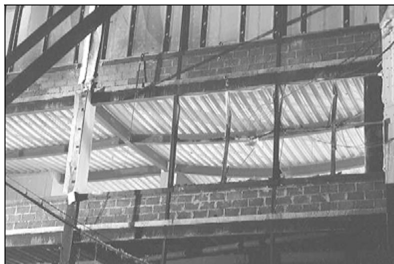
Figure 2.14 Deformed structure during fire
