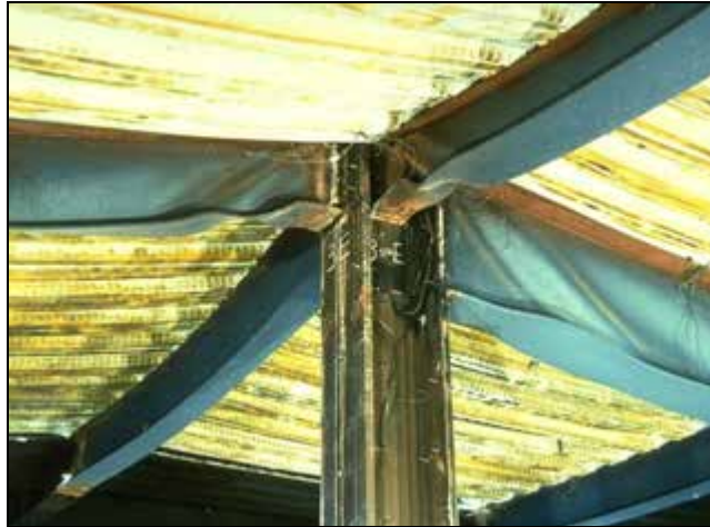
Figure 2.20 Column head showing buckled beams
