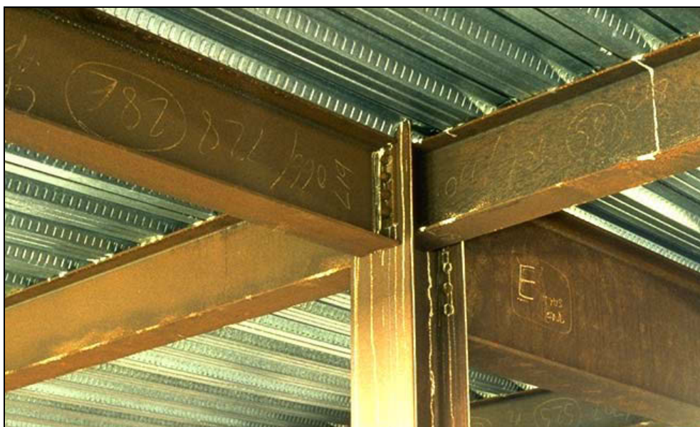
Figure 1-2 View of unprotected steel structure
