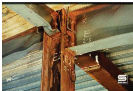
Deformed state of steel members around protected steel column
