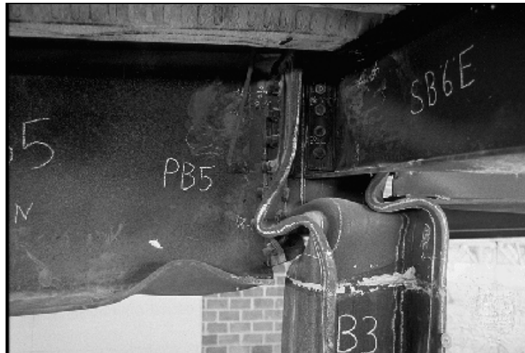
Figure 2.7 Squashed column head following the test
