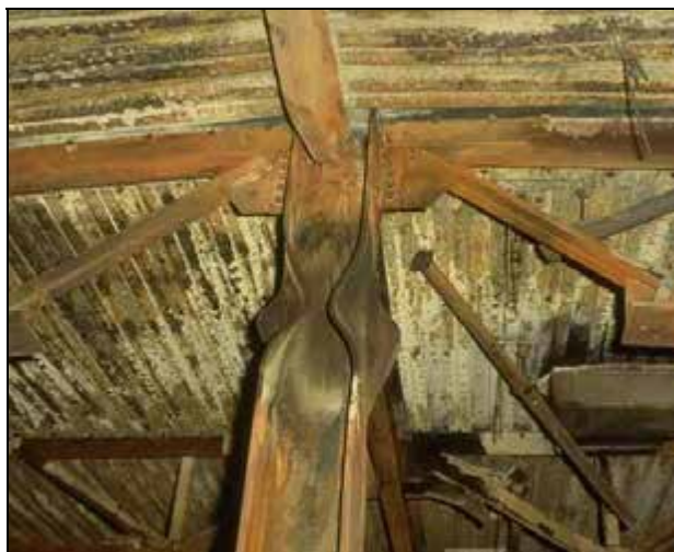
Figure 4.1 Buckled column and deformed beams at Broadgate
