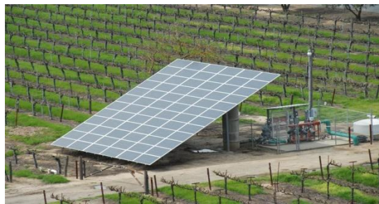
Fig. 5 Photovoltaic panel view and electric generator to provide the pump irrigation water to a vine plantation [203, 204]
