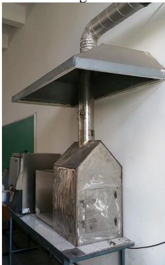
Fig. 7 The new gas collection hood
