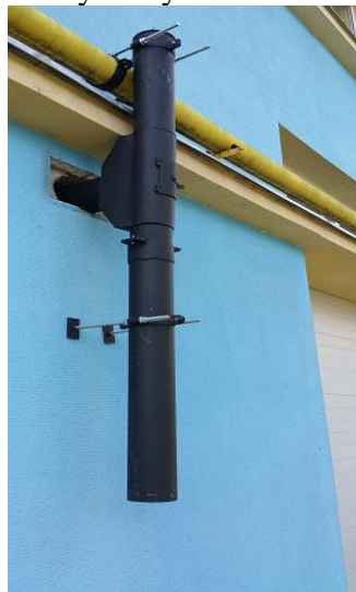
Fig. 8 The gas purification installation
