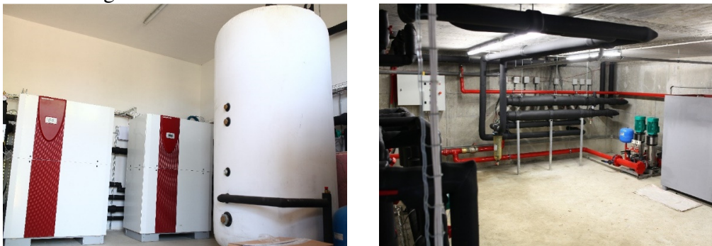
Figure 2 – Heat pumps and boreholes distributor
