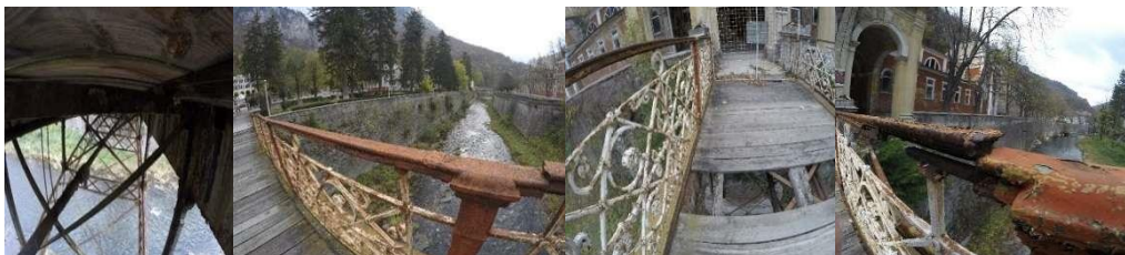
Fig 7. The degree of degradation of the bridge
