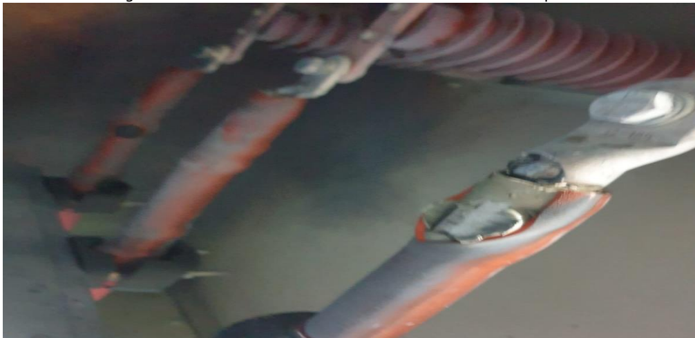
Figure 6.2. 20kV LES terminal end faulted in the 20kV L3-phase.
