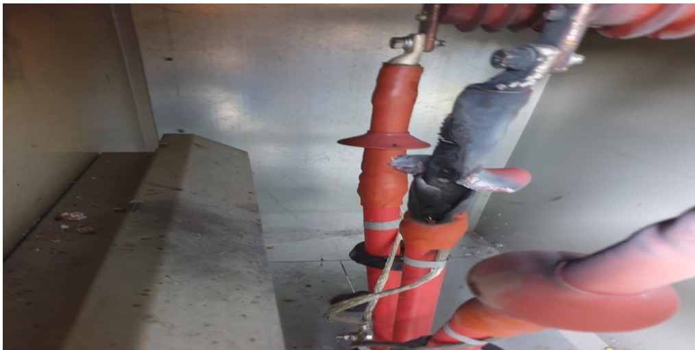
Figure 6.1. 20kV LES terminal end faulted in the 20kV L2-phase.
